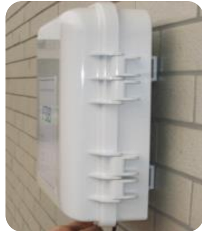
FTTH termination box in the building
