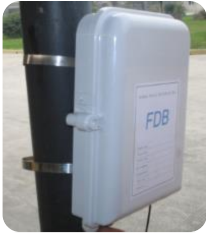
FTTH termination box on the pole
